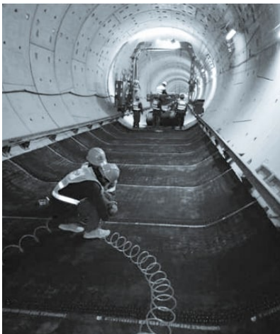
Ballast Mat: Wuhan Metro
